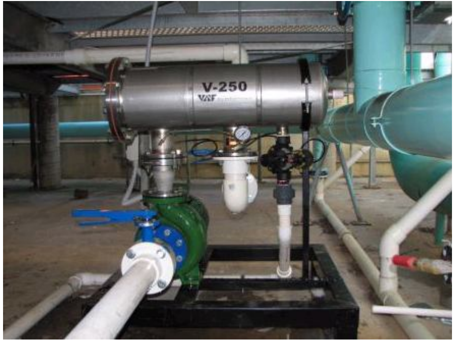
Cooling Tower Water Filtration
