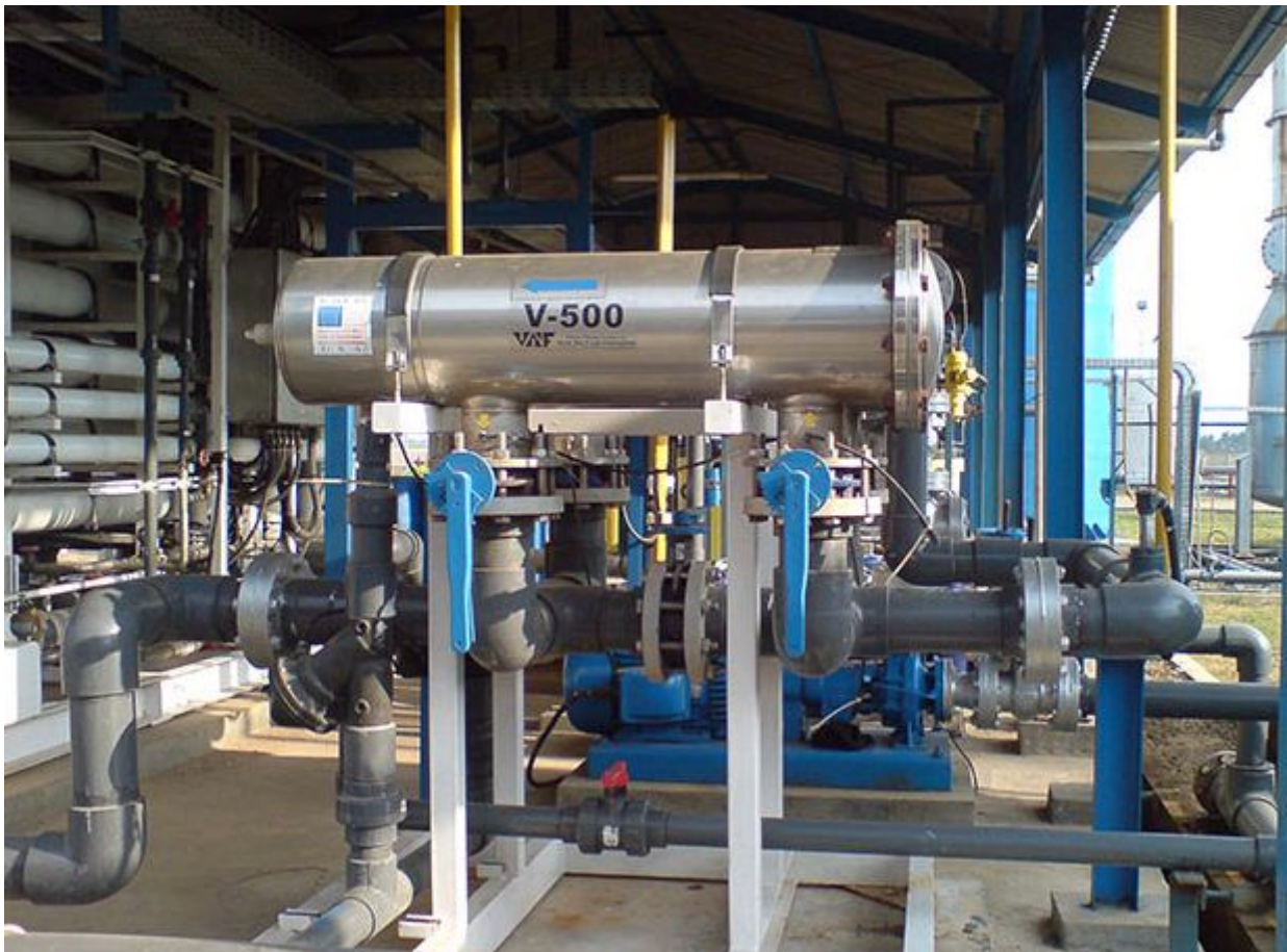
Filter RO for Petroleum Produced Water Reinjection-Pre
