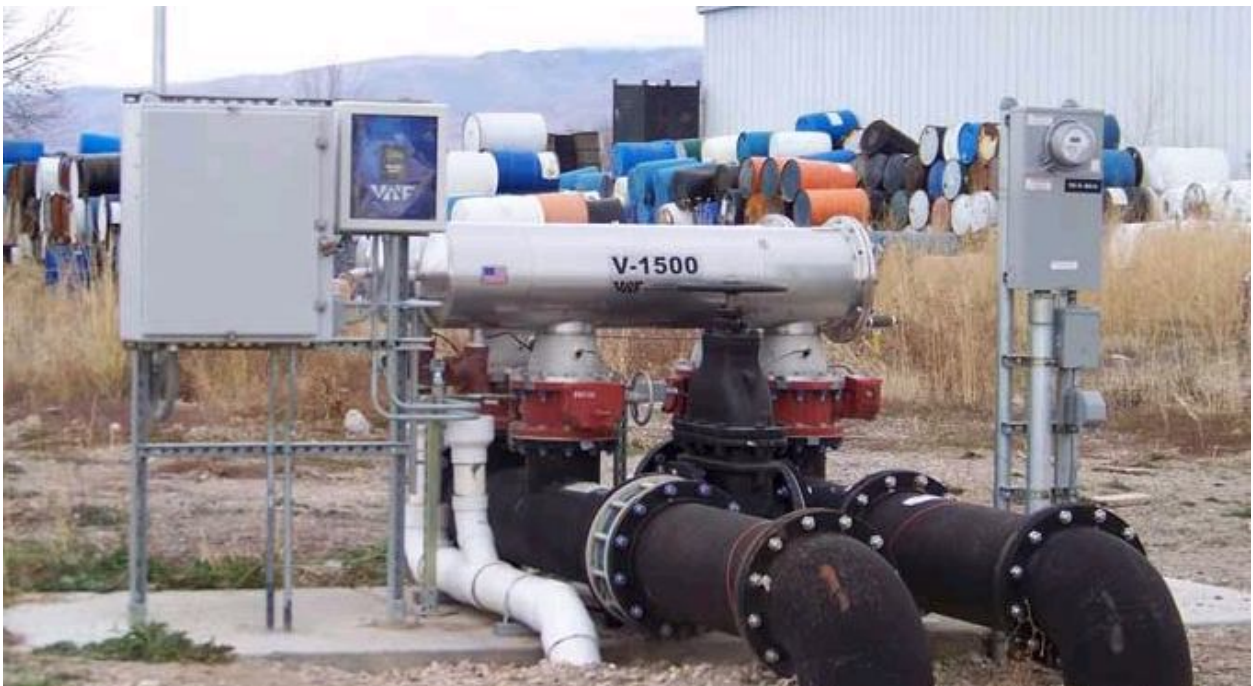
Filter Skid With Bypass Manifold
