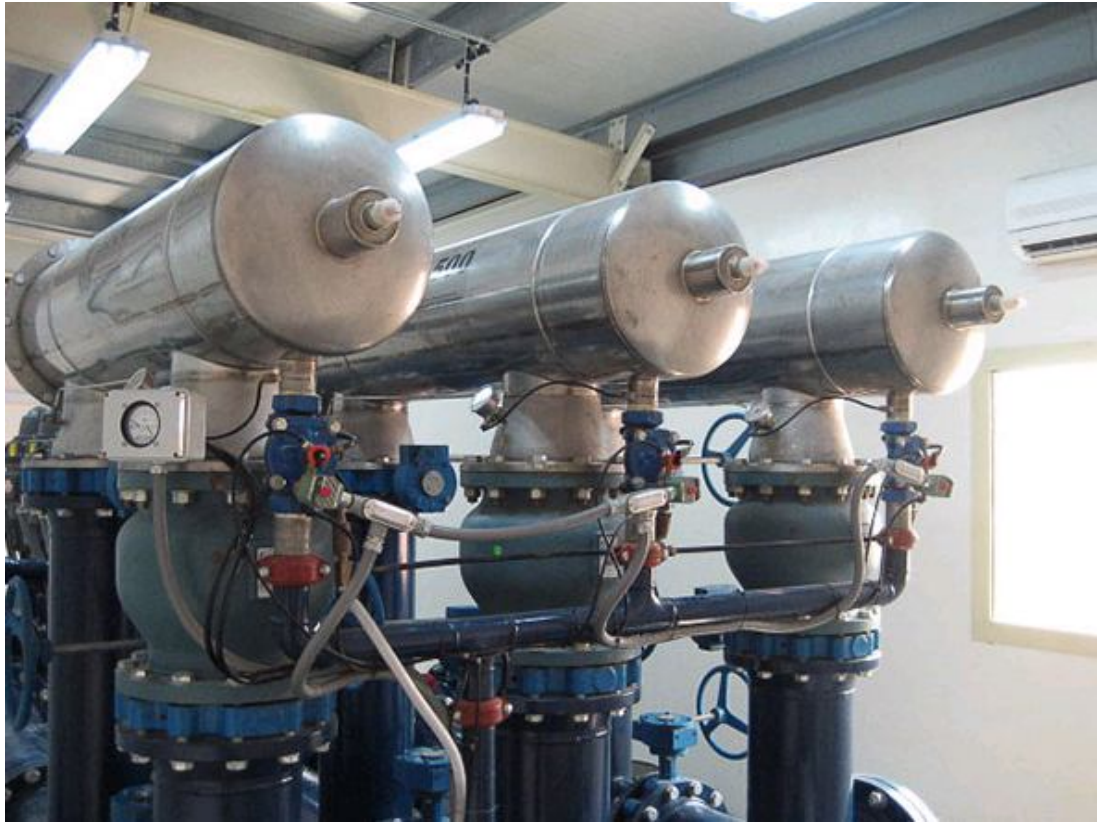
Irrigation Pond Water Filtration
