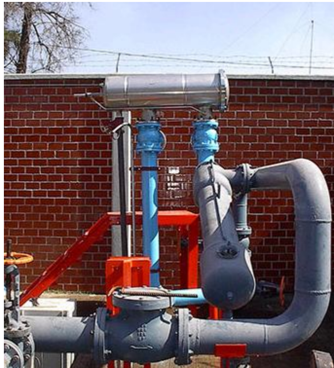
Centrifugal Sand Separators–Cooling Tower Filtration
