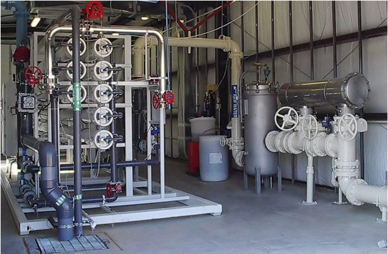
Filtration of Reverse Osmosis-Pre
